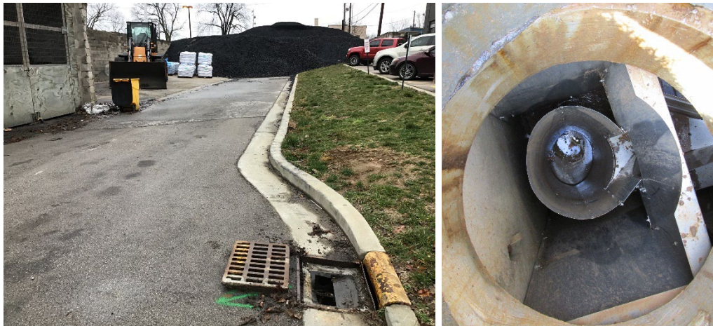
Figure 6.1—Coal Pile BMP HydroKleen® Inlet Filter (left) and Woodland Glenn FloGard® Vortex Separator (right)
