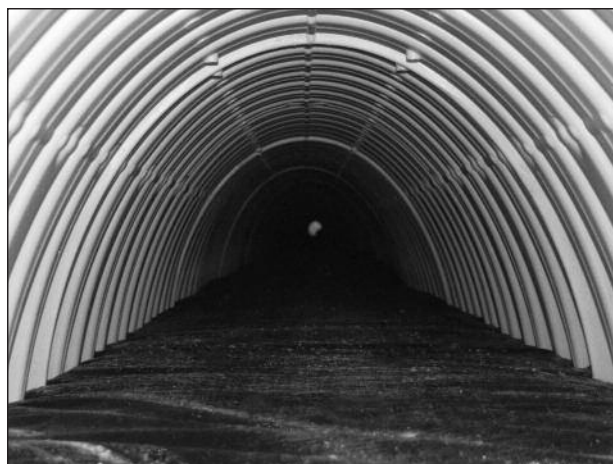
Looking down the Isolator Row.
